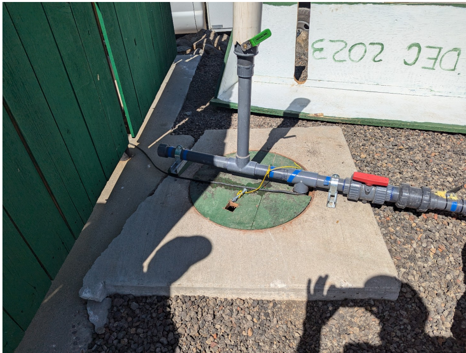
Figure 3: Damaged concrete at Station #1 adjacent to generator and controls slab
